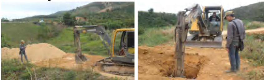
Figure 2.4. Digging soil samples at Dak Noh lake, Dak Nia commune, Gia Nghia town, Dak Nong (Photo taken by PhD student)
